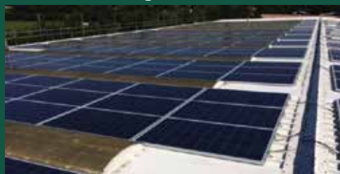
Camlab solar panels cover the entire roof
