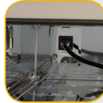
Interior Electrical Outlet
